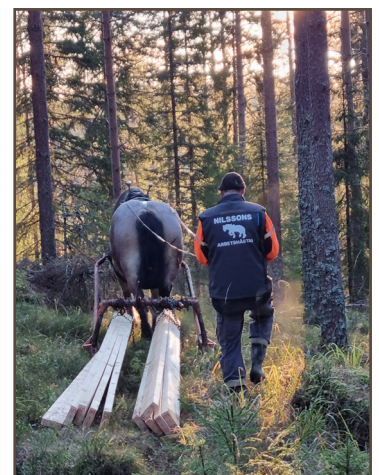
Working horse on Finnvägen again, but this time for laying out duck boards.
